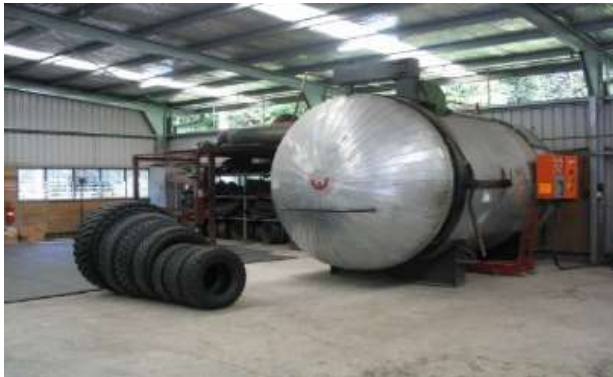
Tyre retreading plant, Timika
